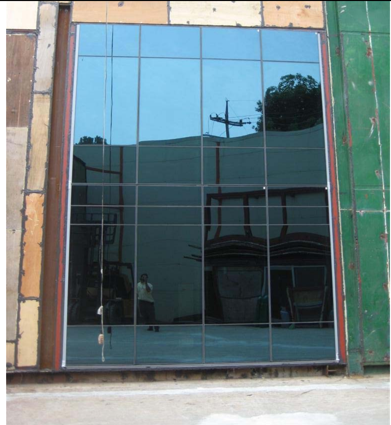
EN-WALL Songdo City Mockup Installed at CNC Testing Laboratory Seoul, South Korea
